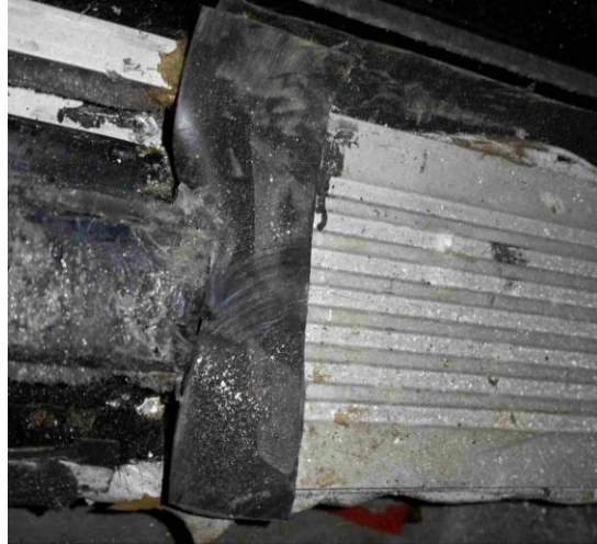
Figure 20 – Rubber gasket on sill at threshold ends on the exterior
