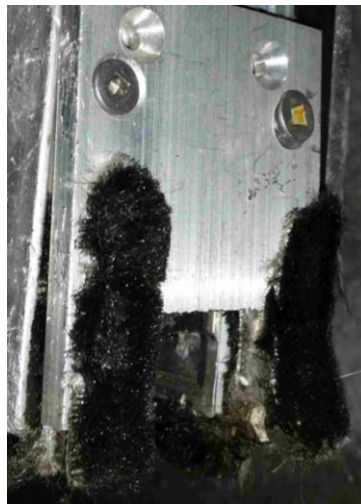
Figure 18 – Aluminum plate on sash bottom
